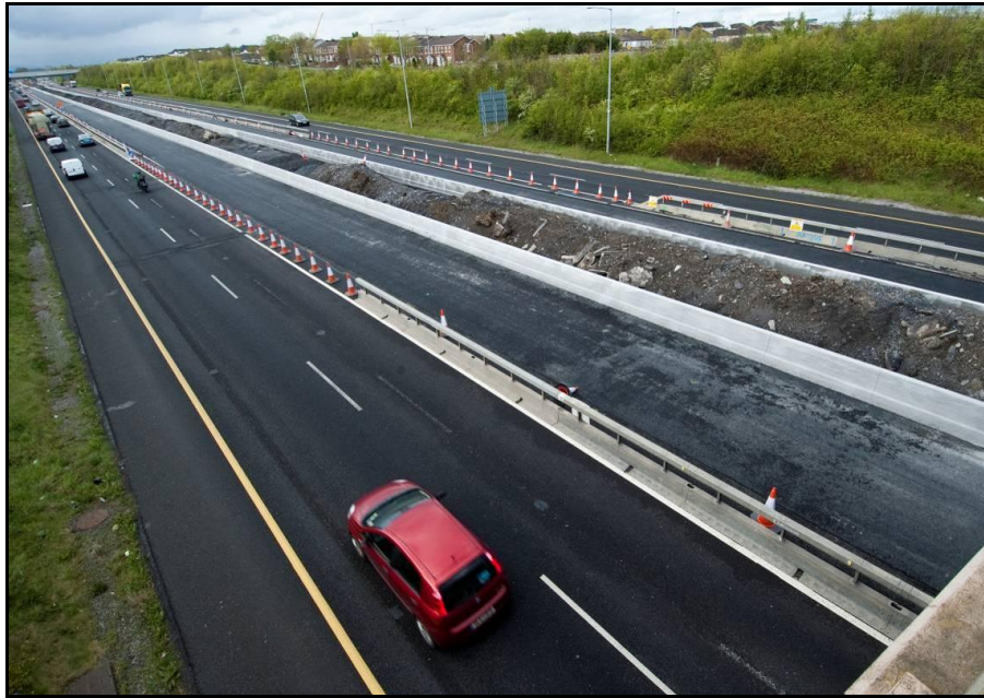
Plate 12.7: M1 Widening under construction – highlighting traffic management and maintenance of two running lanes in both directions during a later stage in construction.
