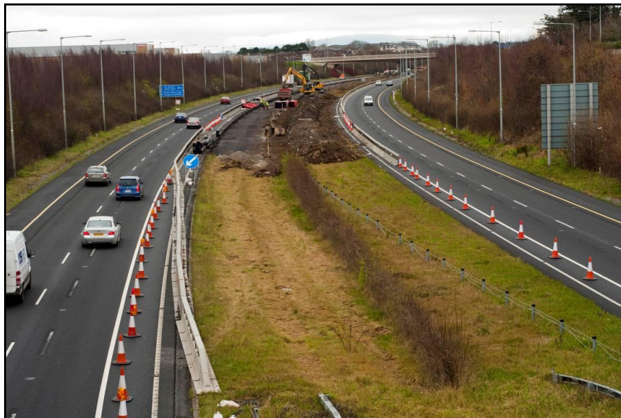
Plate 12.6: M1 Widening under construction – highlighting traffic management and maintenance of two running lanes in both directions.
